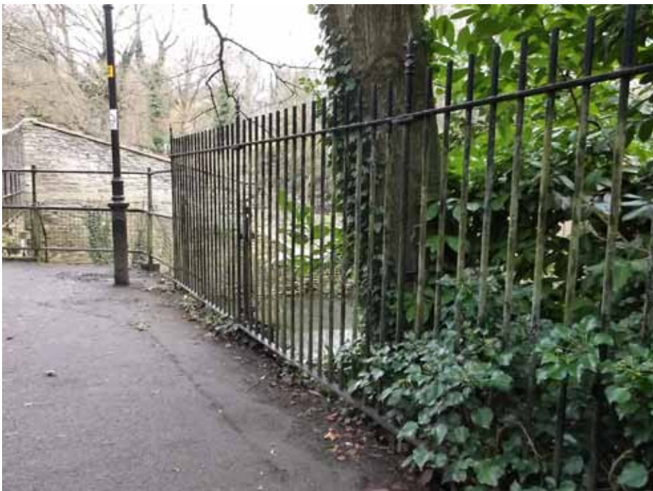
2. The Abbey House garden railings extend from the top of the steps to the bridge. The appearance would be improved by the removal of green algae.
