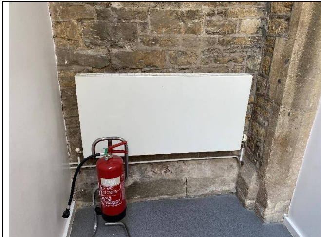
Figure 12: Example of wall mounted hot water radiator
