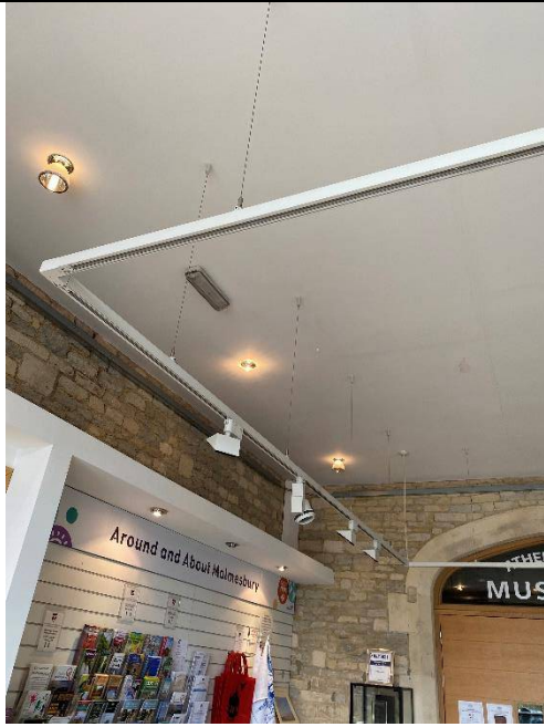
Figure 23: Typical lighting in main areas
