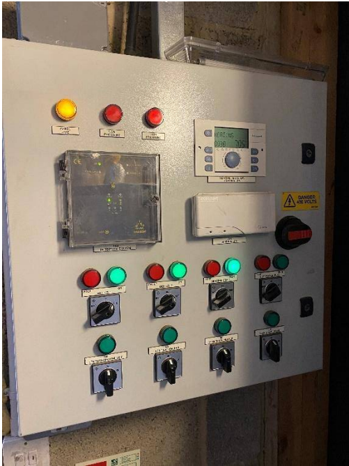
Figure 14: Honeywell heating controls
