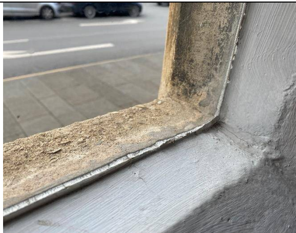
Figure 21: Close-up showing single glazed pane
