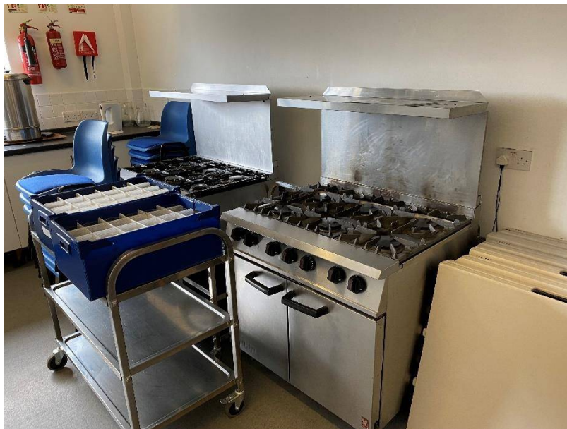
Figure 40: Existing gas fired appliances considered for replacement
