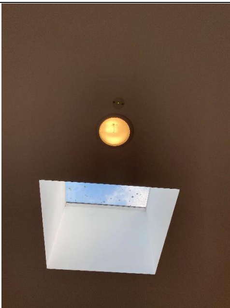
Figure 25: Skylights providing passive lighting in corridors along with a halogen light fitting
