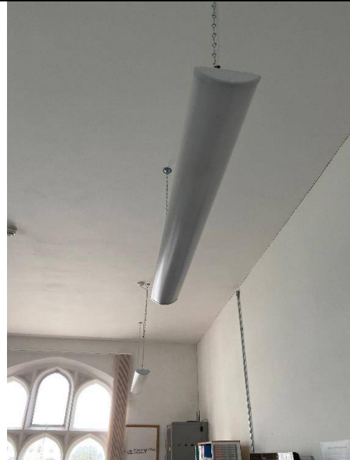
Figure 24: LED lighting in main office
