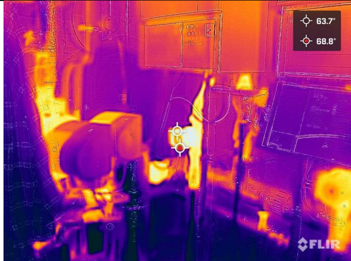
Figure 11: Thermal image of uninsulated pipework
