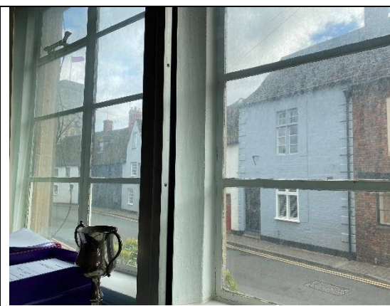
Figure 32: Example of retrofit double-glazed interior windows to reduce heat loss
